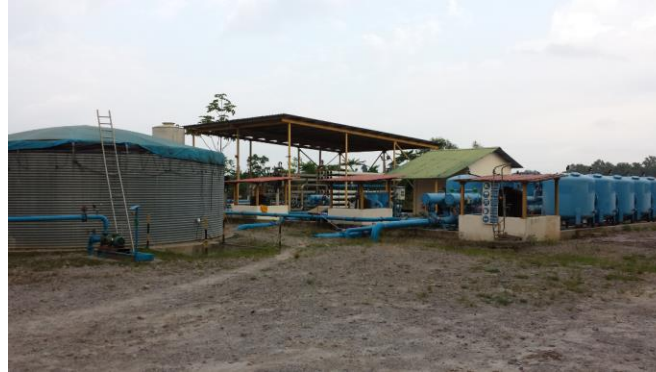
Improper Equipment & Controls
