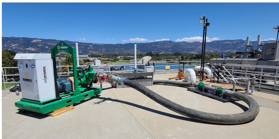
Temporary installation at GSD for the trial period.
